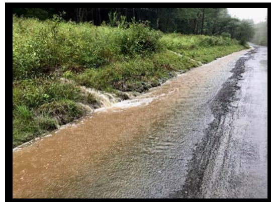
Hurricane Ida storm event. Underdrain and cross pipes keeping water from topping over the road.
