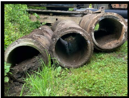
Old concrete pipe that was full of sediment replaced with a plastic pipe.
