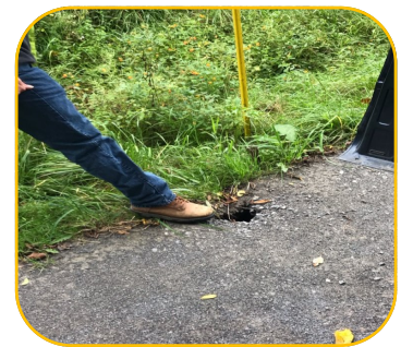
Culvert failing, leaving hole in road
