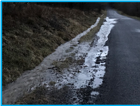
Cross pipe failing. Water out on road turning into ice.
