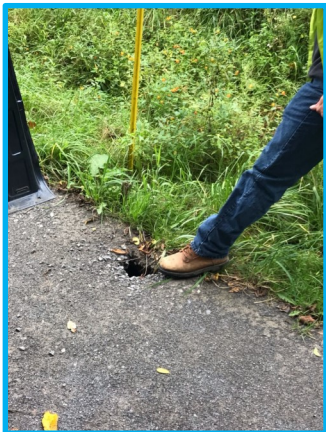
Before—pot hole at outlet of pipe in road surface
