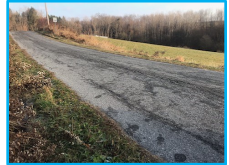
Before—road surface cracking
